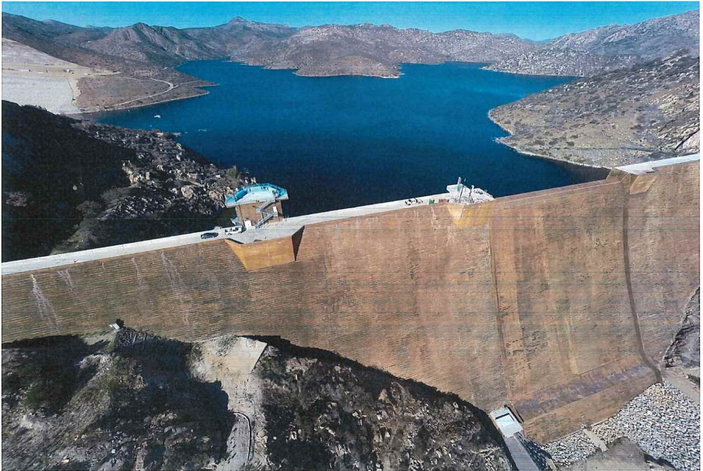
A December 2014 aerial view of the San Vicente Dam and reservoir. (John Gibbins/San Diego Union-Tribune)
