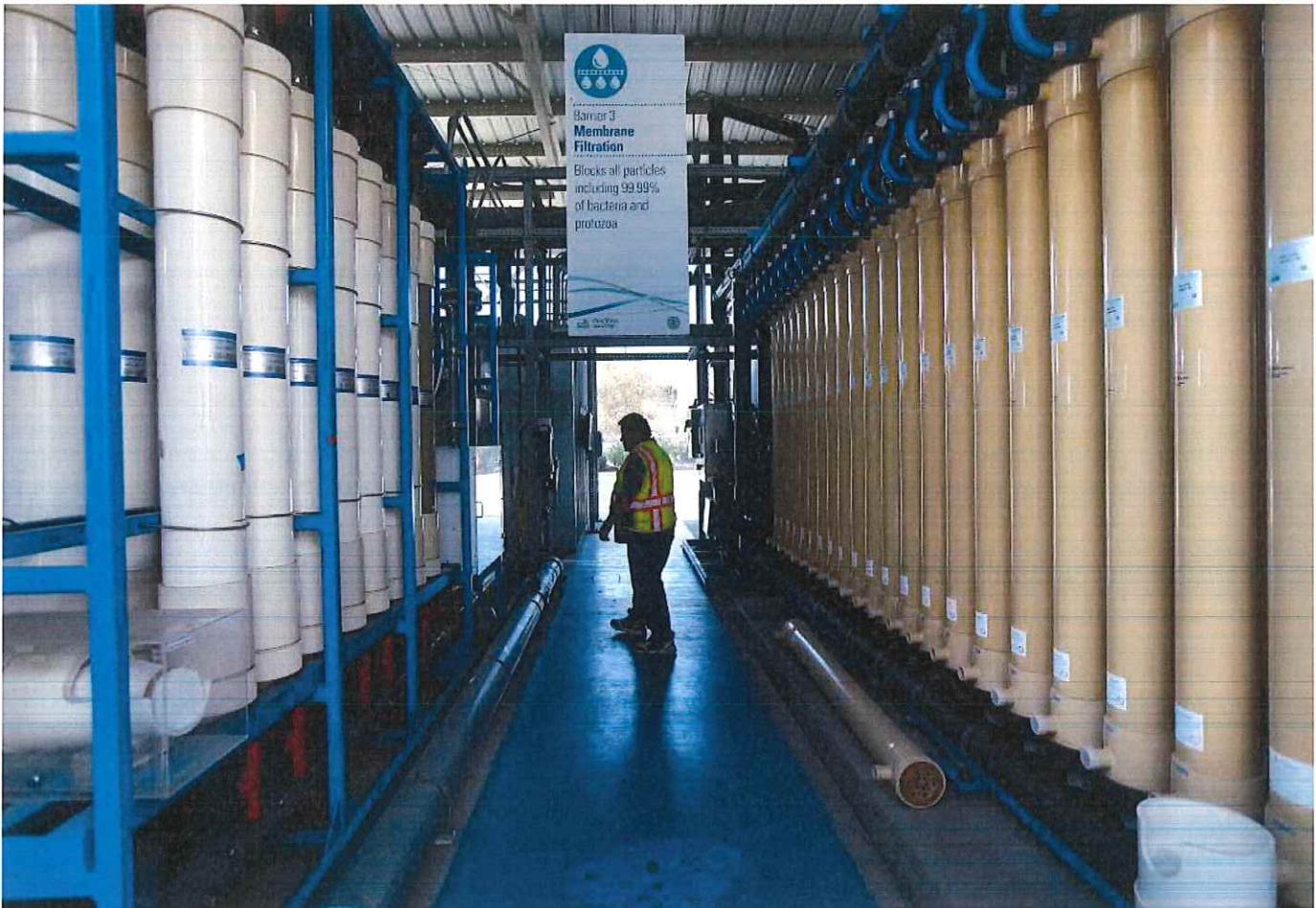
A supervisor walks through the membrane filtration columns at the Pure Water Demonstration Facility in San Diego. (K.C. Alfred/The San Diego Union-Tribune)
