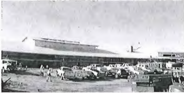
Highland Community News photo by Charles Roberts — East Valley Water District new headquarters building is a hub of activity on Thursday morning and crowds of workers move toward a Feb. 14 opening date.
